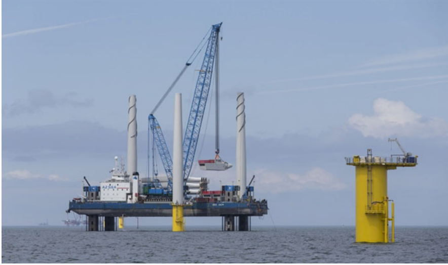
Fig. 19.1 A2SEAs SEA JACK during the construction of the Gwynt y Mor wind farm. Image Source: A2SEA (2016)
